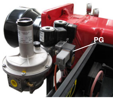
Fig. 17 - Gas pressure switch
